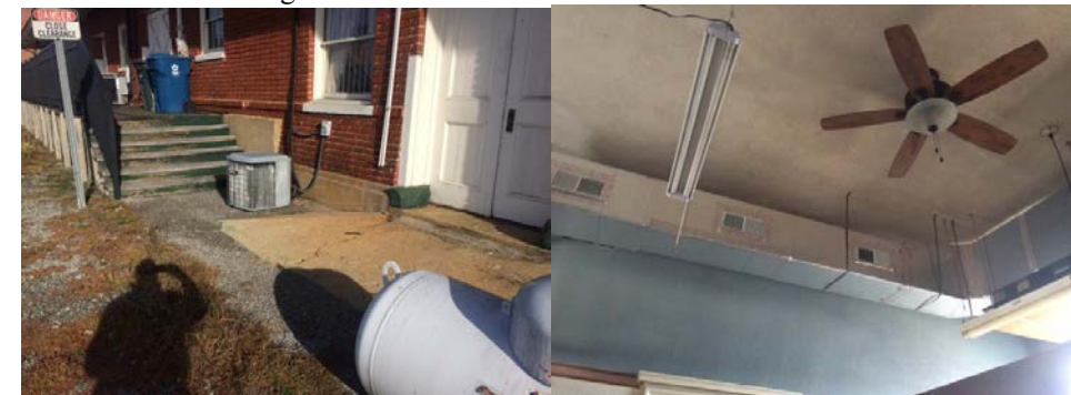
Antique Shop Condenser Unit
