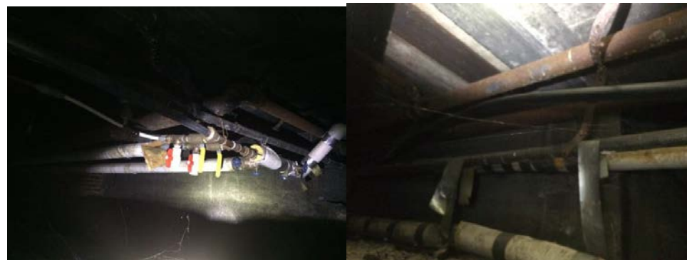
Domestic plumbing in basement
