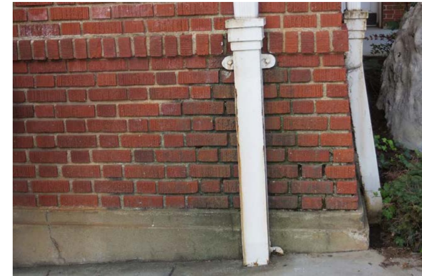
5. Mortar Erosion at NE Corner Downspouts
