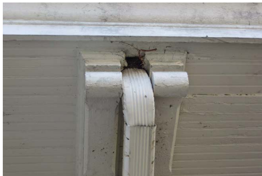
4. Water Damaged Overhang Soffit with Bad Downspout Connection at Internal Gutter
