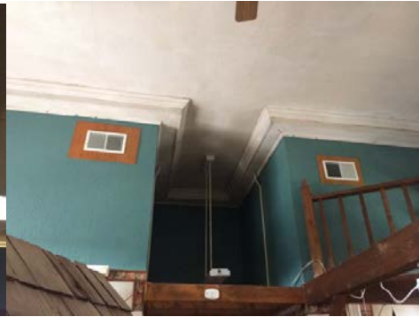
Diffusers in other room of antique shop
