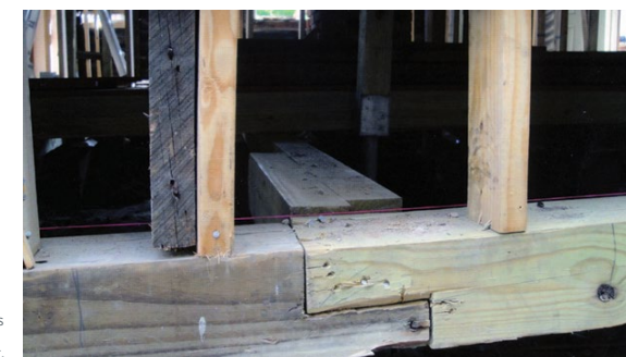
[33] Retaining as much as possible of the historic wood sill plate and replacing only the termite-damaged wood is always the preferred and recommended treatment.
