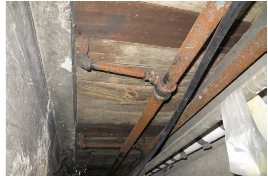
9. Pipe Trench Wood Plank Failure
