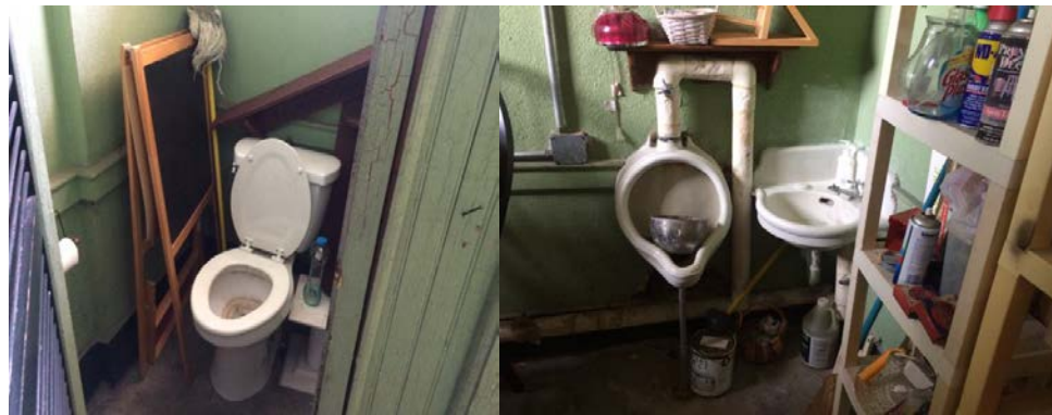
Plumbing and plumbing fixtures in antique shop
