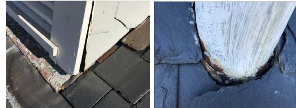
Rusted Vent Pipe & Step Flashing
