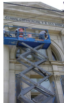
[1] An alkaline-based product is appropriate to use to clean historic marble because it will not damage the marble, which is acid sensitive.
