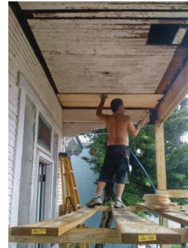
[24] Rotted boards in the beaded-board porch ceiling are being replaced with new matching beaded board.
