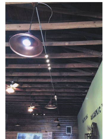
[40] Not Recommended: Removing a finished ceiling and leaving the structure exposed in a historic retail space does not meet the Standards for Rehabilitation.
