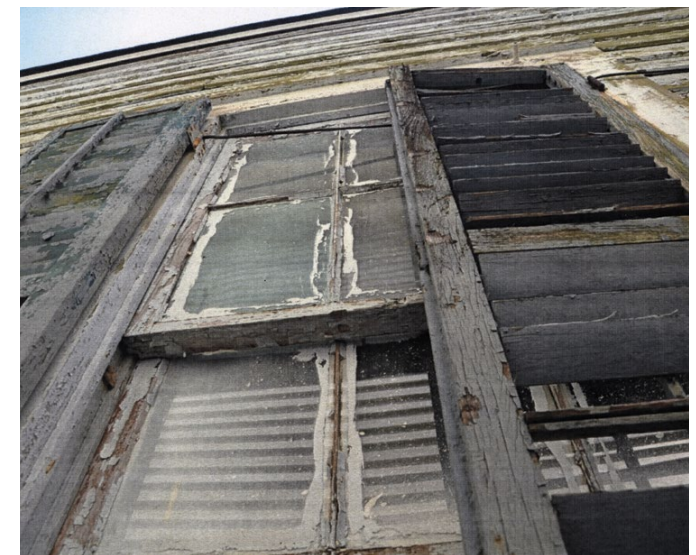
[11] Old and brittle glazing putty should be removed carefully before reputtying to keep window glazing weathertight.
