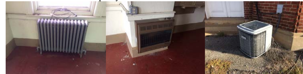
Ticket Office Radiator
