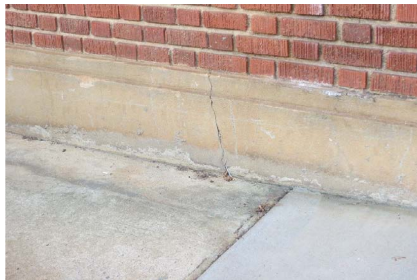
8. Typical Foundation Wall Crack at East End
